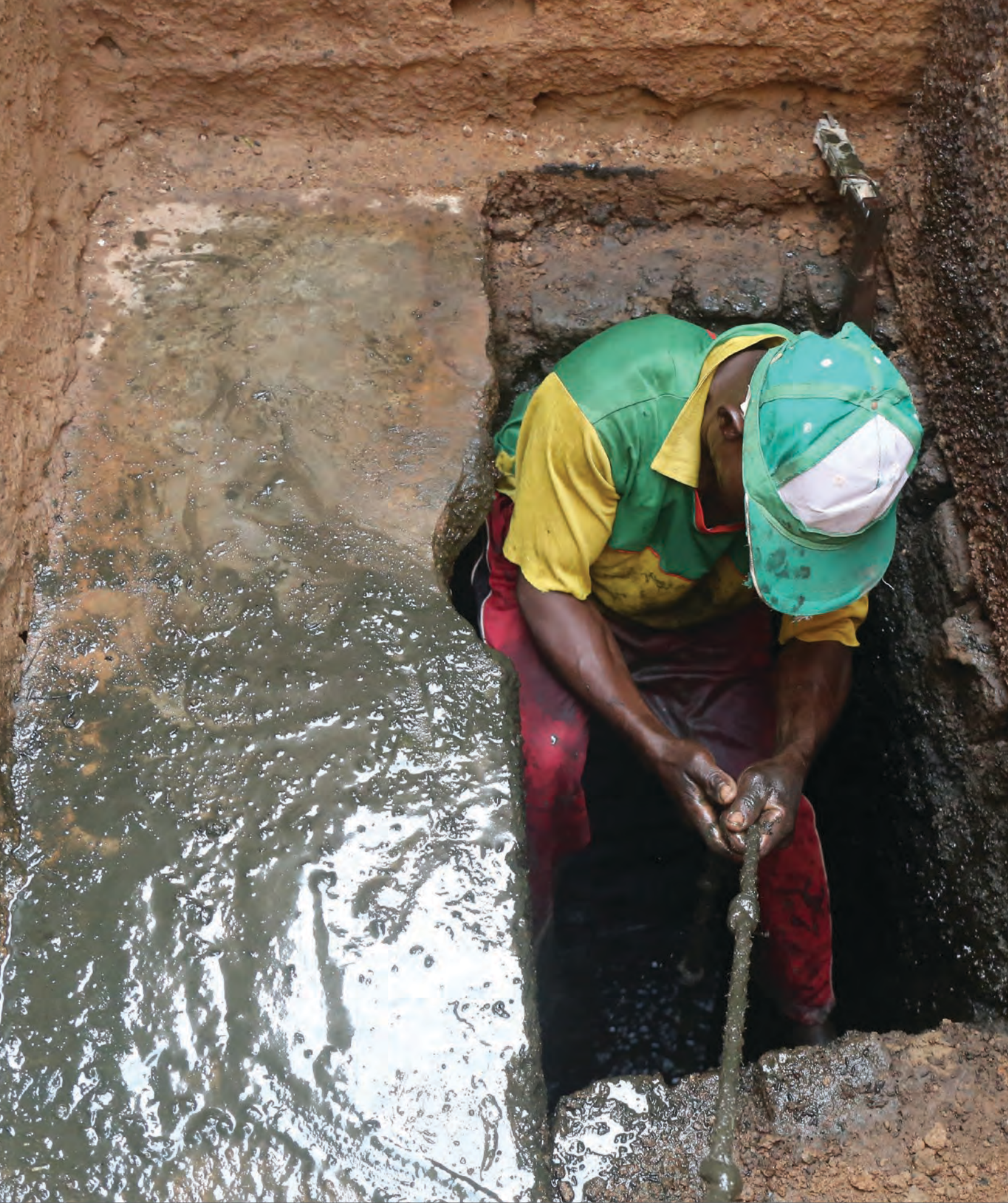
Wendgoundi Sawadogo, 45, manual emptier, entering the pit of a latrine with a rope, Ouagadougou, Burkina Faso, July 2019. © WaterAid / Basile Ouedraogo. Used with permission. Permission required for reuse.
